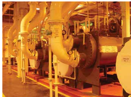
Central Chiller Plants
