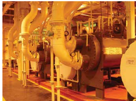
Central Chiller Plants
